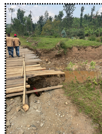
Image: Bridge damaged by floods in Rwanda | Scottish Fair Trade
